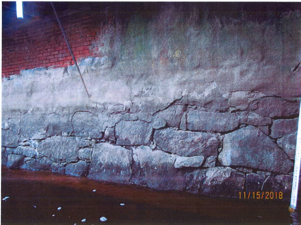
Photo 16: Wingwalls - Northeast wingwall: Typical scattered hollow areas of shotcrete.
