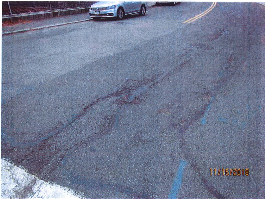
Photo 7: Wearing Surface - Eastbound lane: Heavy wear with typical scattered cracks, some sealed.
