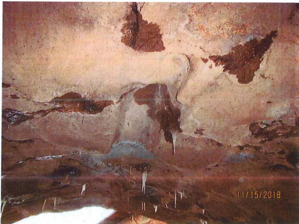
Photo 12: Keystone Area - 3ft south of north fascia: Area of missing keystones with shotcrete filling voids.
