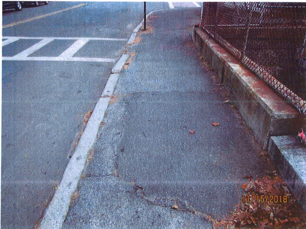
Photo 8: Sidewalks - South sidewalk: Scattered areas of delamination and cracking.
