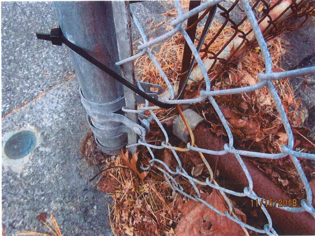
Photo 9: Railing - Northwest corner: Detached bottom rail with zip ties holding chain link fence to rail post.
