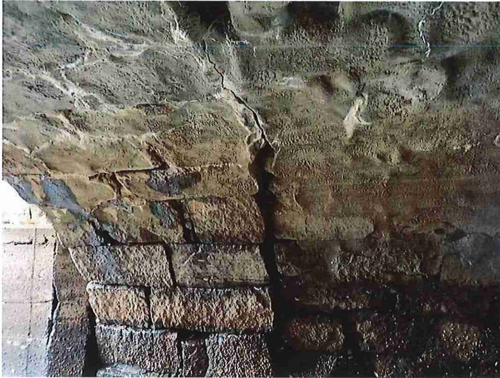
Photo 3: Void above the west spring line at 7' in from the south fascia.
