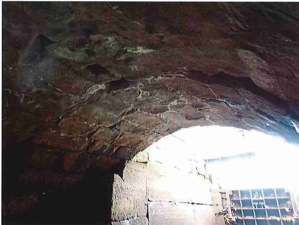
Photo 2: Full length crack in the arch at 7' in from the south fascia and voids in the keystone area.
