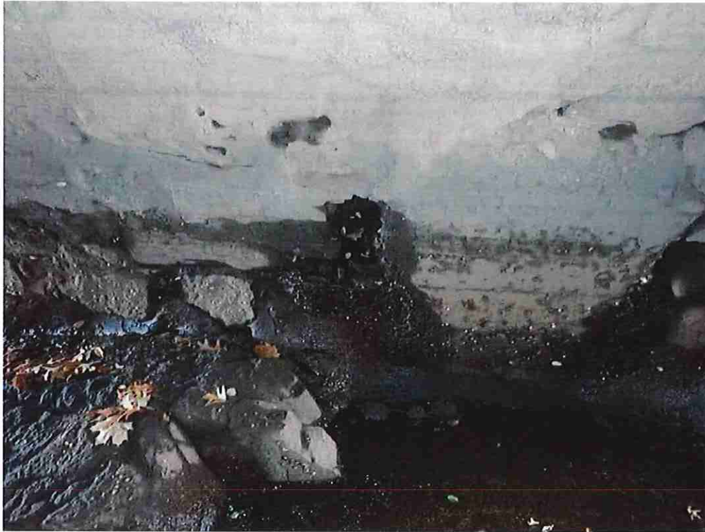
Photo 1: Void in the arch at 18' in from the north fascia, 3-1/2' above the west spring line.
