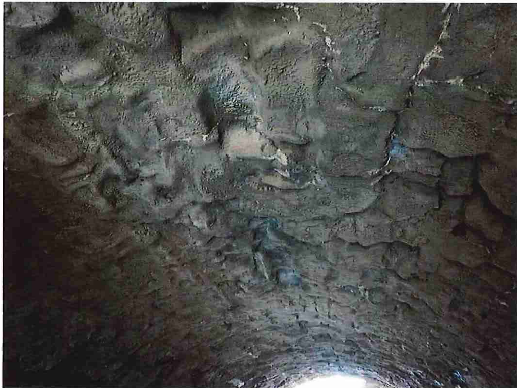
Photo 4: Typical voids and unevenness throughout the keystone area.
