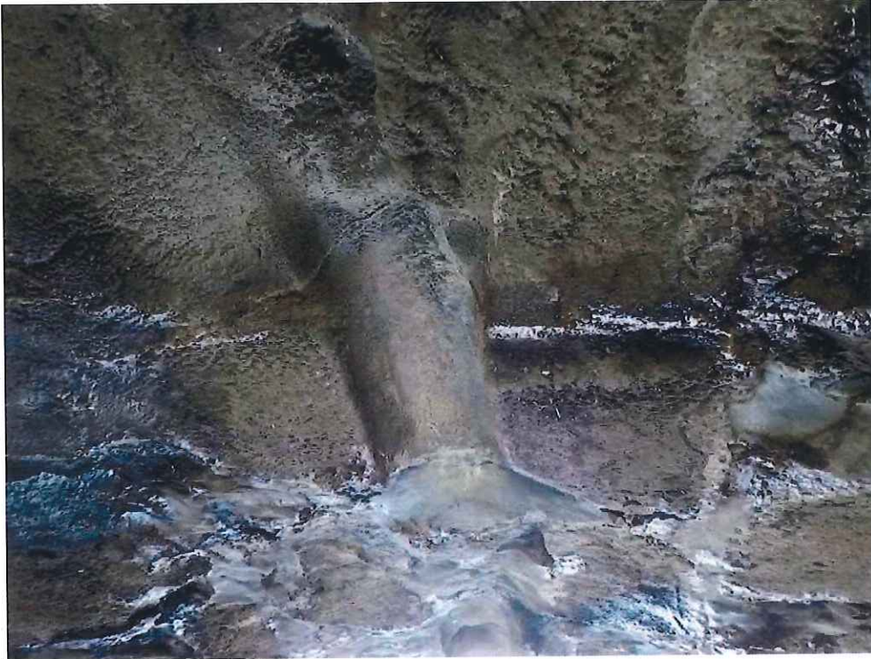
Photo 17: Keystone Area - 7'-0" from North Fascia: Missing keystones resulting in a 3'-0" long x 9" wide x 6" deep void.
