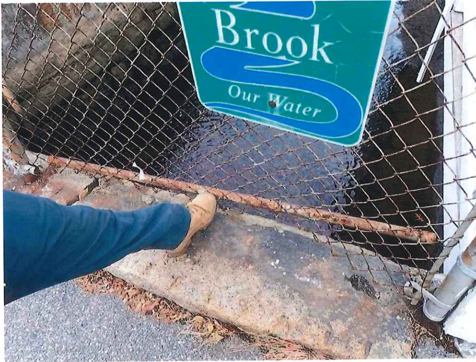
Photo 9: North Elevation Bridge Railing - Northeast Panel: The bottom railing is detached from the receivers and hangs loosely.
