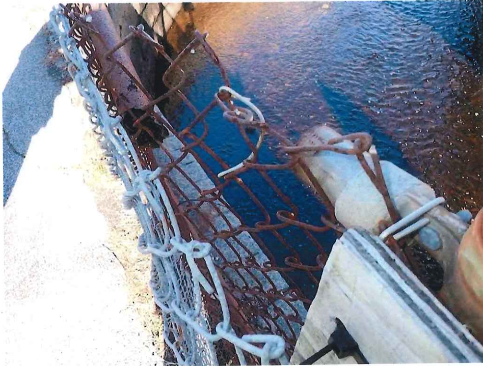
Photo 13: NW Retaining Wall Railing - 6th Panel from South Corner: At the 5th post from the south corner, the top rail has 100% section loss resulting in it being detached from the post and hanging loosely.
