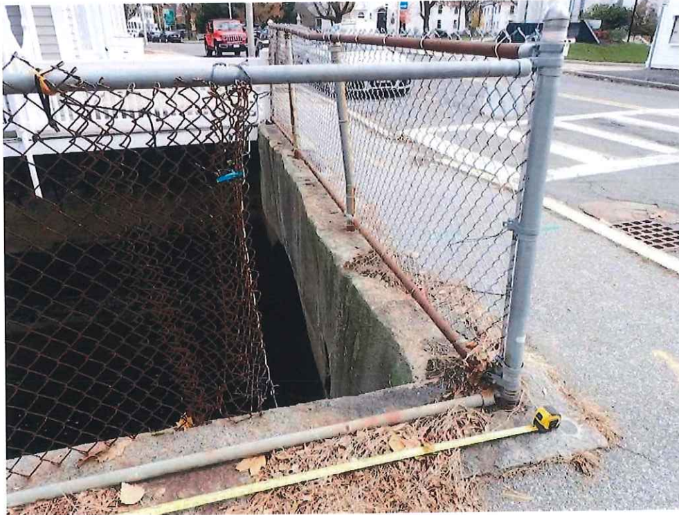
Photo 10: NW Retaining Wall Railing - South Corner: The chain link fabric was unsecured along bottom rail for 6'-0" and disconnected from top rail and corner post for 2'-8" L resulting in a fall hazard of approx. 9 feet.
