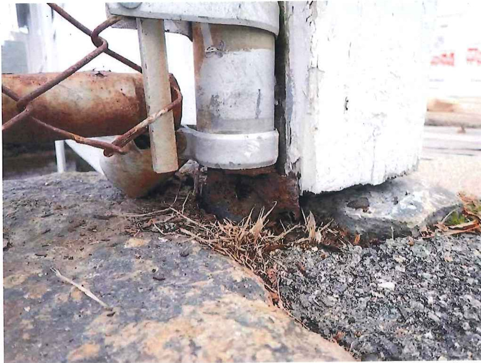
Photo 8: North Elevation Bridge Railing - East Corner: Section loss resulting in the post being detached at its base. Post is otherwise secured to adjacent property's wooden fence post with tension bands.
