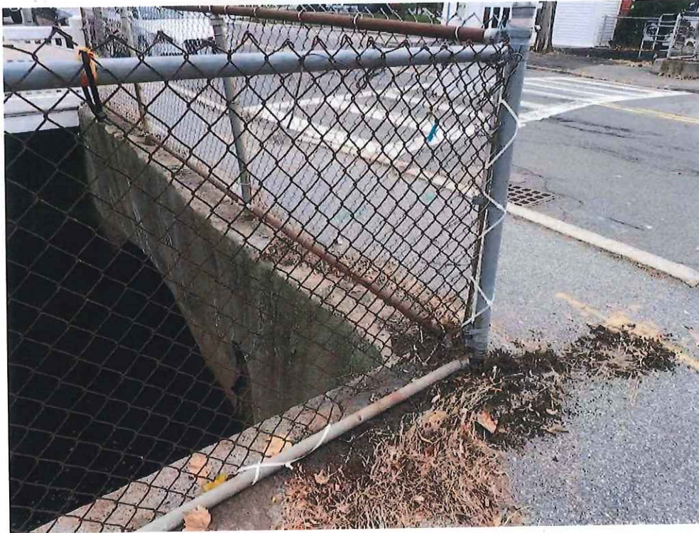
Photo 11: NW Retaining Wall Railing - South Corner: Supplemental zip ties were installed by inspectors to secure chain link fabric. Four (4) zip ties total.
