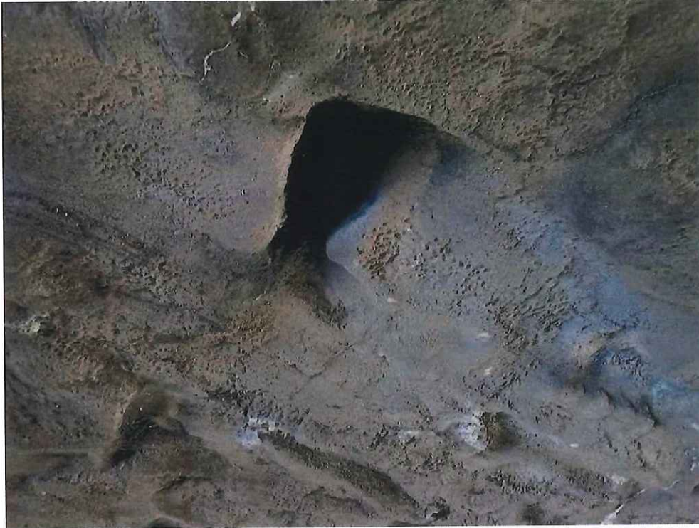
Photo 19: Keystone Area - 18'-0" from North Fascia: Missing keystones resulting in a 6" long x 12" wide x 9" deep void.
