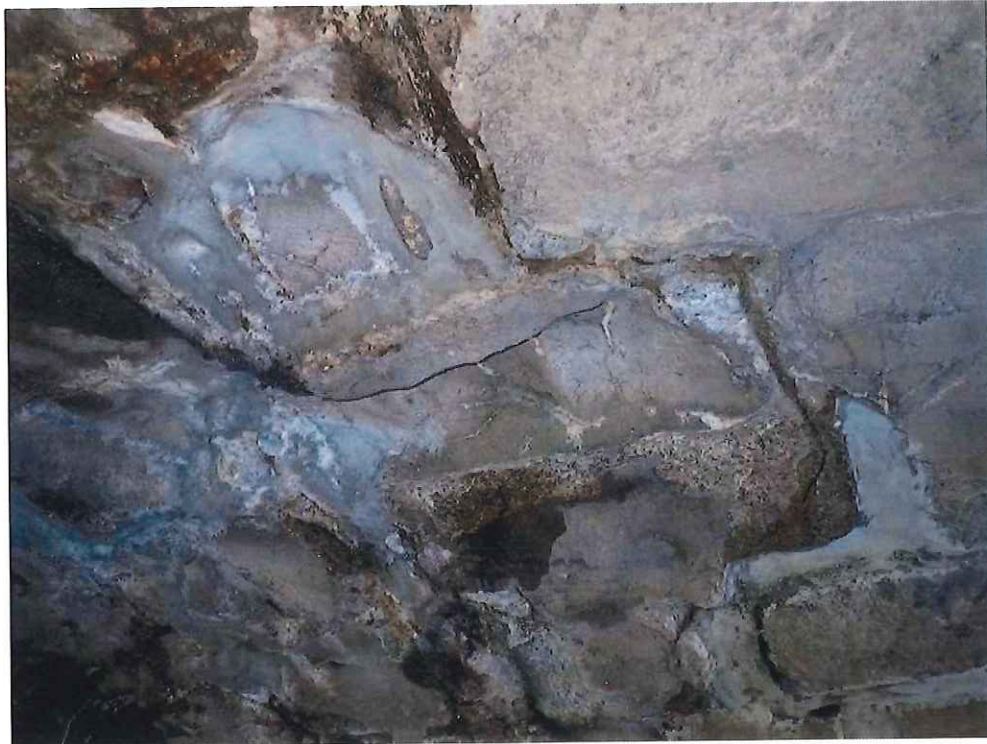
Photo 16: Keystone Area - 2'-6" from North Fascia: Missing keystones resulting in a 2'-0" long x 9" wide x 6" deep void.
