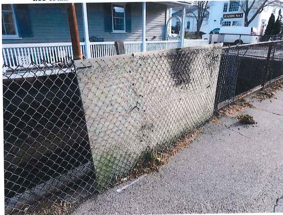
Photo 12: NW Retaining Wall Railing - 5th Panel from South Corner: The Posts and panel are very loose and movable by hand. The panels consists of a plywood board and supplemental chain link fabric.
