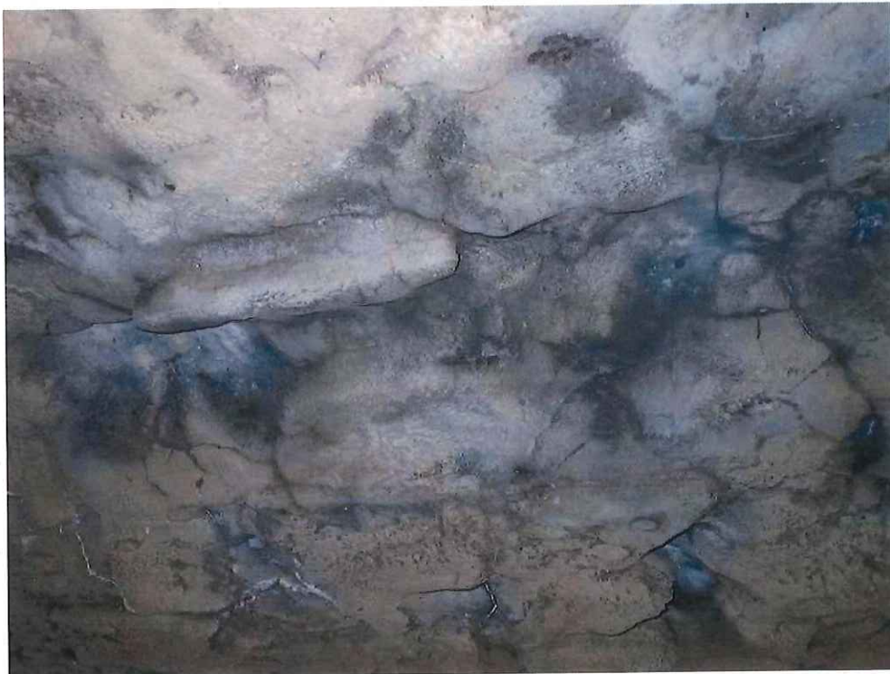
Photo 20: Keystone Area - 22'-0" from North Fascia: Missing keystones resulting in a 5'-0" long x 12" wide x 6" deep void.
