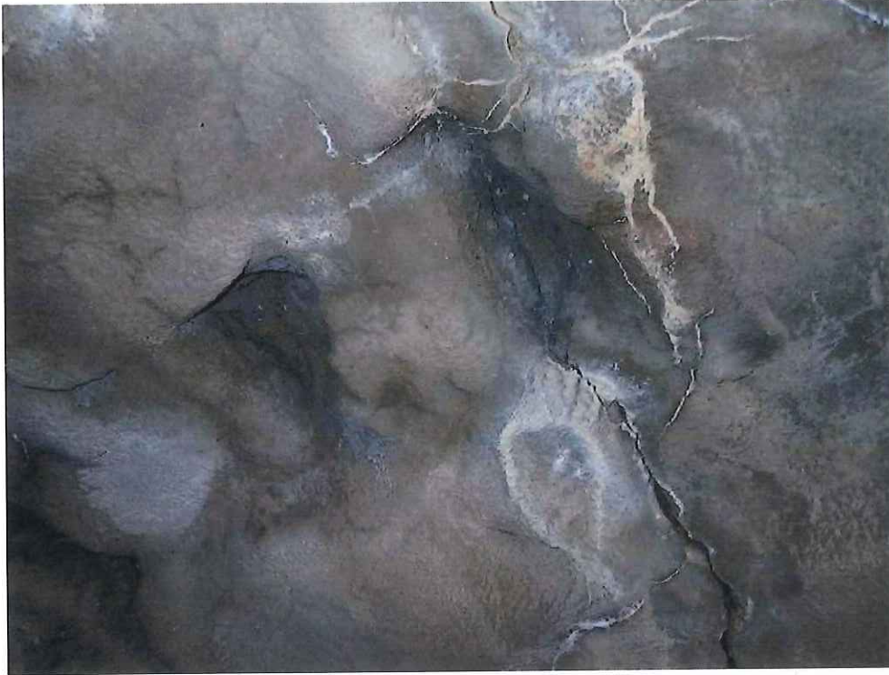
Photo 21: Keystone Area - 35'-0" from North Fascia: Two missing keystones resulting in an up to 7" long x 11" wide x 8" deep void.
