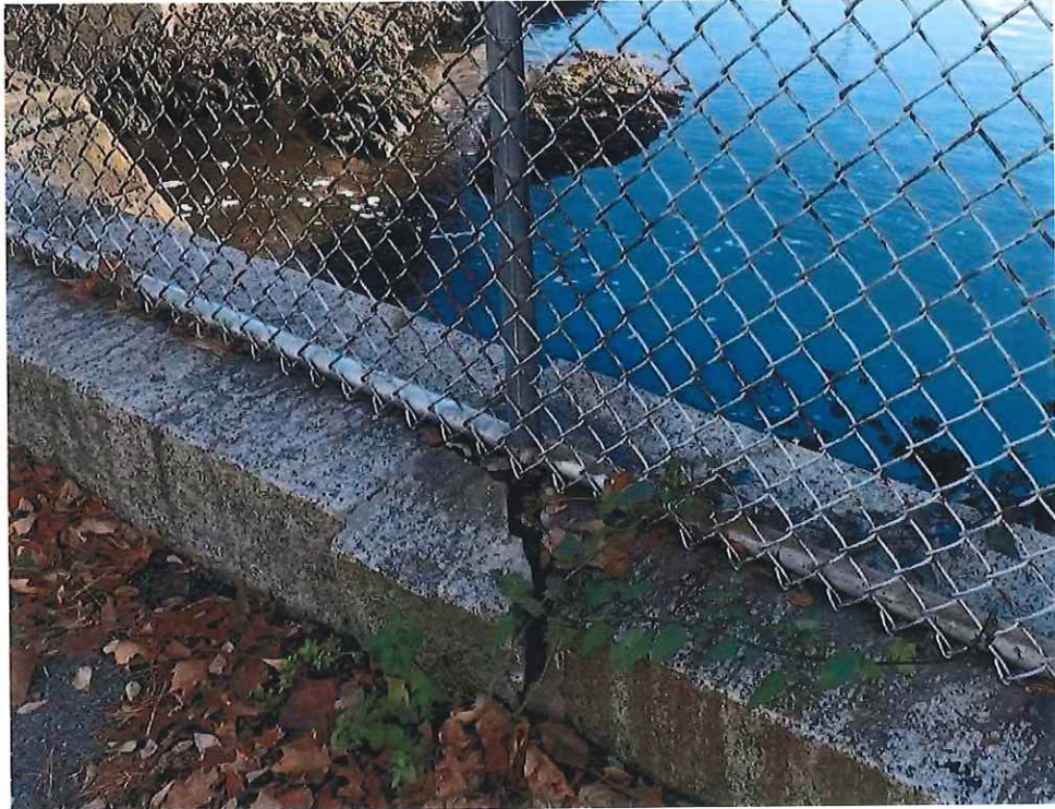
Photo 15: SW Wingwall Railing: The granite rail base is cracked at the 3rd post west of the bridge. Post is loose and appears detached within the base.
