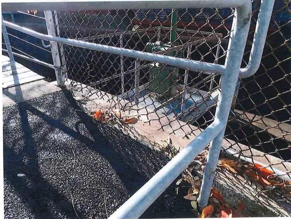
Photo 14: SE Wingwall Railing - 2nd Panel from North: The panel has no bottom rail and there is a gap between the chain link fabric and the top of the wingwall.
