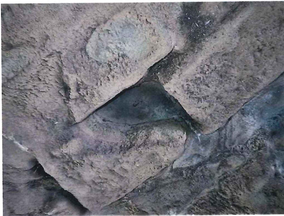
Photo 18: Keystone Area - 14'-0" from North Fascia: Missing keystones resulting in a 12" long x 9" wide x 6" deep void. Stones around void settled up to 6".
