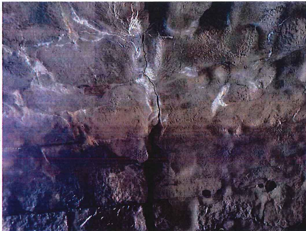
Photo 14: Arch/Arch ring - 7'-0" north of south fascia: Shotcrete ends at west spring line resulting in exposed masonry with a void 4" w x 2'-8" deep.
