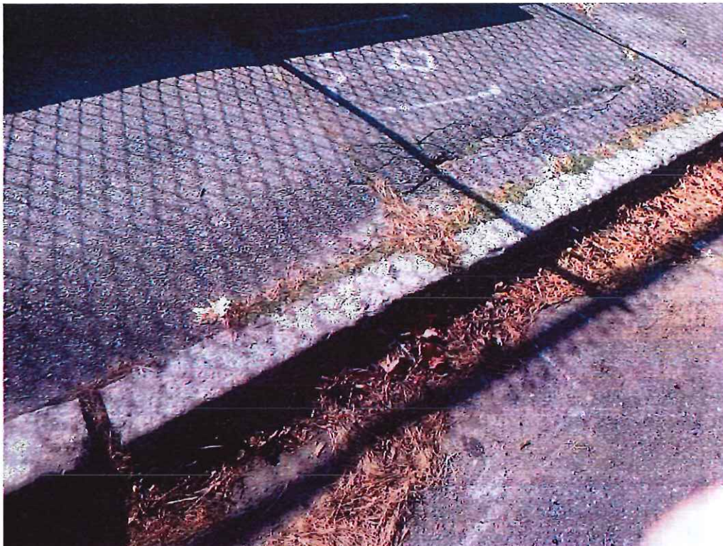
Photo 8: Sidewalks - South Sidewalk: Area of cracks up to 1-1/2" wide.
