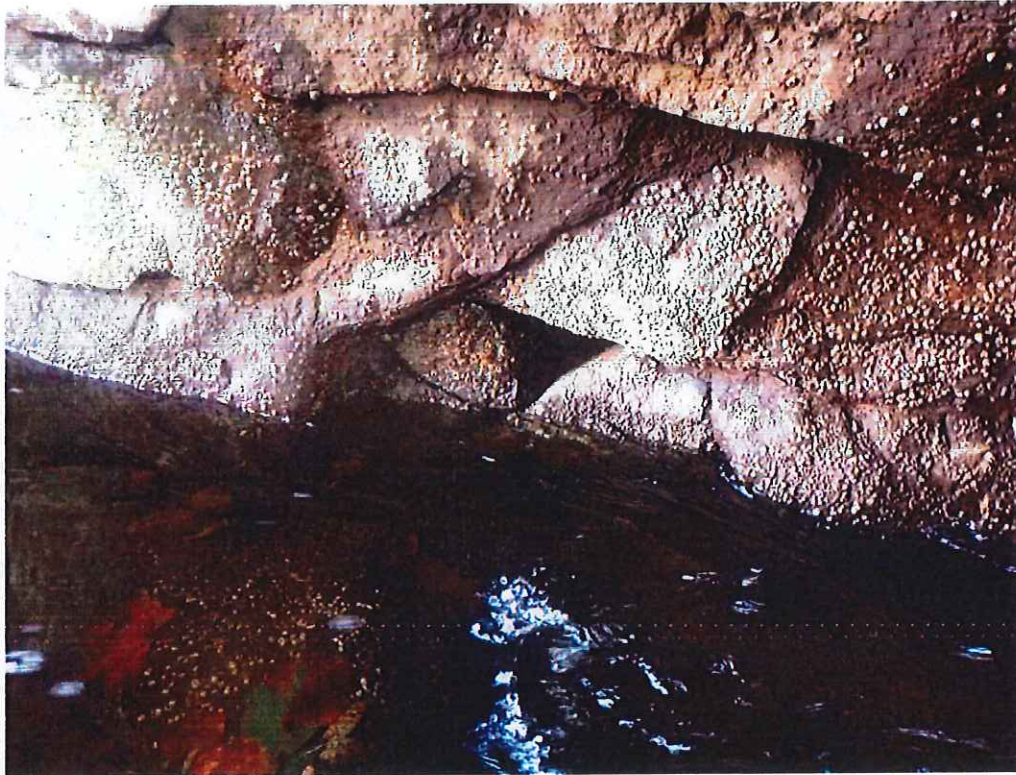
Photo 21: Spring Line - 9'-0" south of north fascia: East spring line with a void 24" wide x 10" high x 10" deep due to missing stone.
