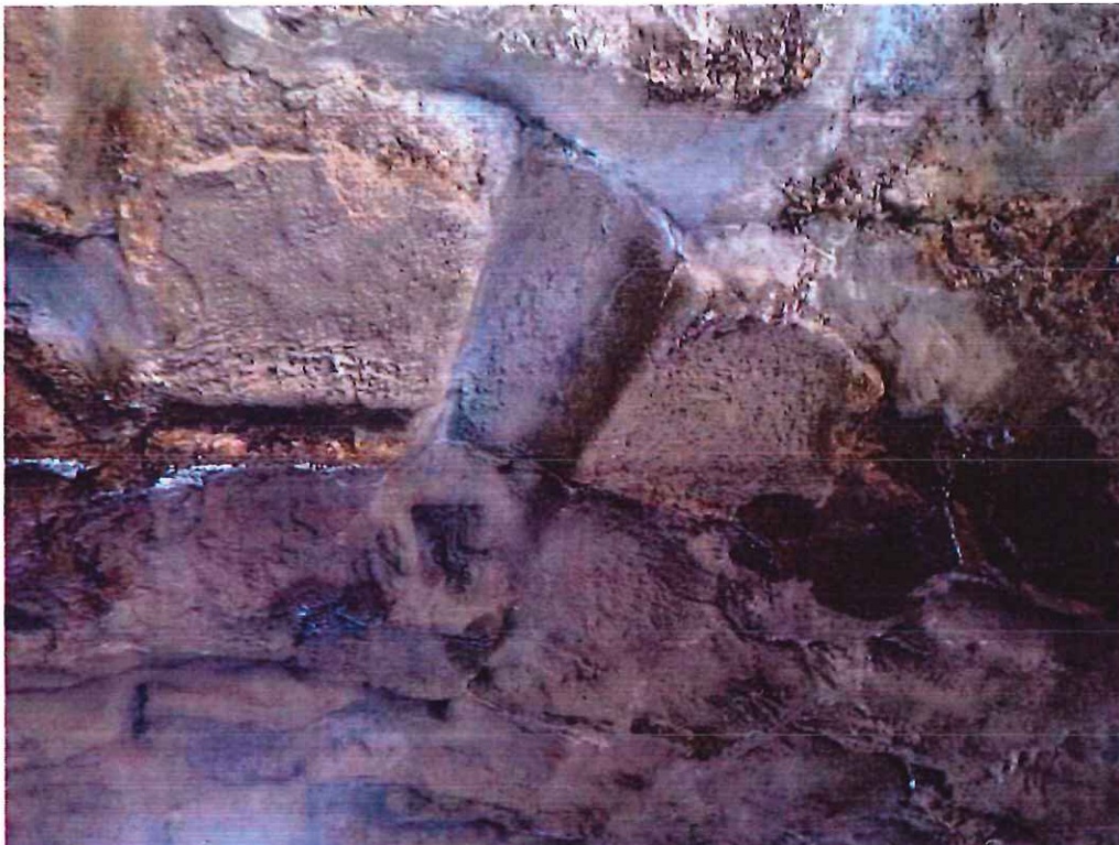
Photo 16: Keystone Area - 7'-0" from north fascia: Missing keystones resulting in a 3'-0" long x 9" wide x 6" deep void.
