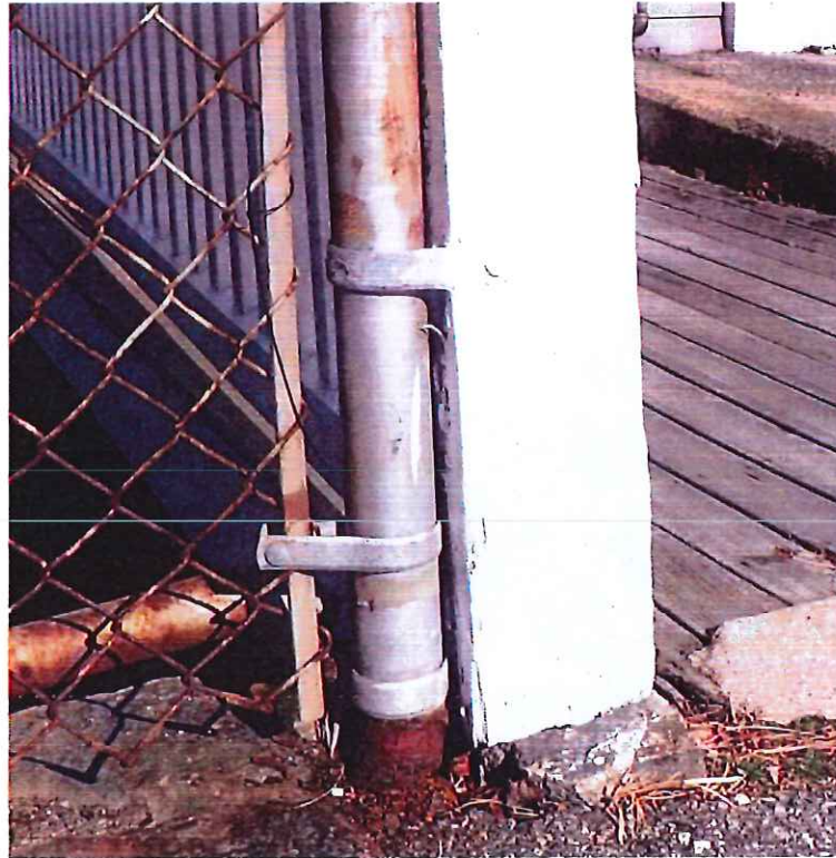
Photo 11: Railing - Northeast Corner: Post is detached at its base and secured only to the adjacent property's wooden post.
