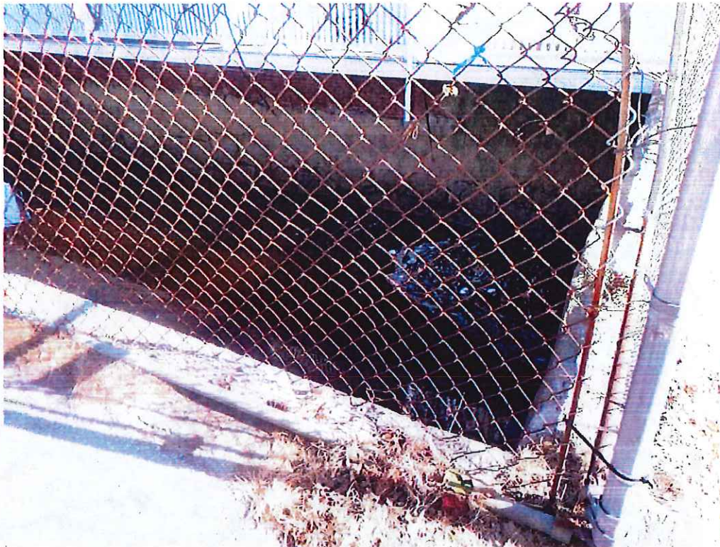
Photo 10: Railing - Northwest Corner: Chain link fabric is unsecured along bottom rail for 5'-0" length resulting in a potential gap and fall hazard.
