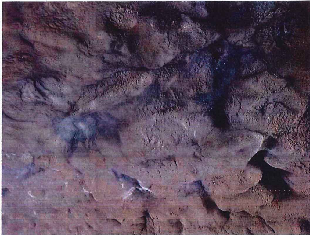
Photo 17: Keystone Area - 22'-0" from north fascia: Missing keystones resulting in a 5'-0" long 12" wide x 6" deep void.
