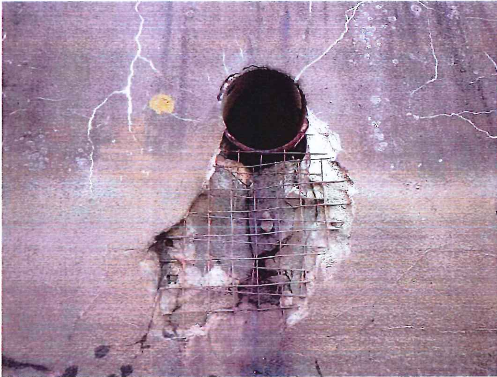
Photo 19: Spandrel Walls - West side of north wall: Spall in shotcrete under drain pipe, 2'-0" wide x 2'-0" high x 3-1/2" deep with exposed wire mesh.
