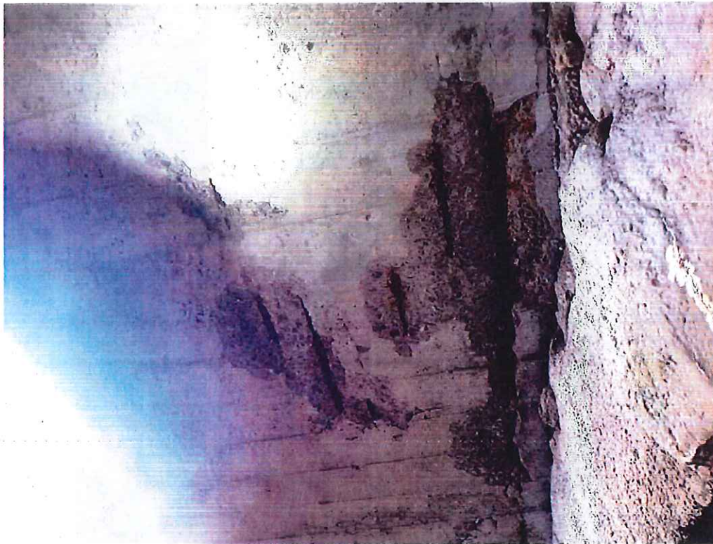
Photo 9: Sidewalks - Underside of South Sidewalk: Widespread deminalation, spalling, and exposed reinforcement. Spalling up to 8'-6" long x 15" wide x 1-1/2" deep adjacent to spandrel wall.
