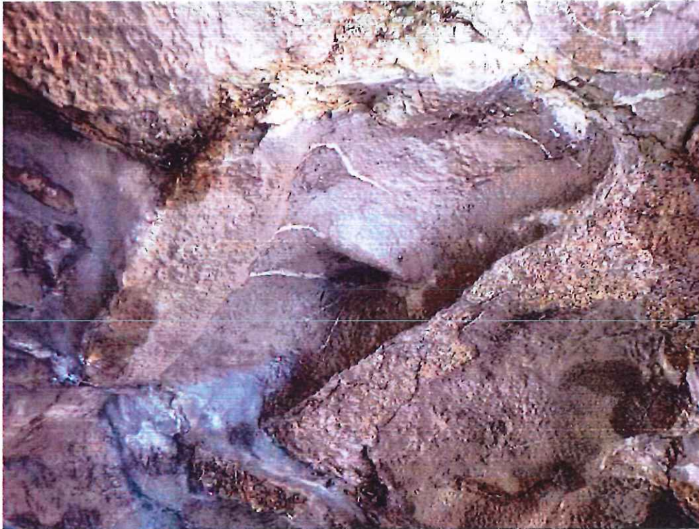
Photo 15: Keystone Area - 2'-6" from north fascia: Missing keystones resulting in a 2'-0" long x 9" wide x 6" deep void.
