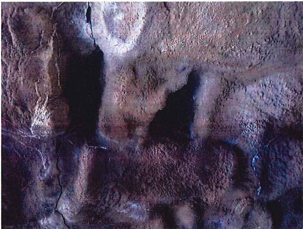
Photo 18: Keystone Area: 35'-0" from north fascia: Two missing keystones resulting in voids up to 7" long x 11" wide x 8" deep.
