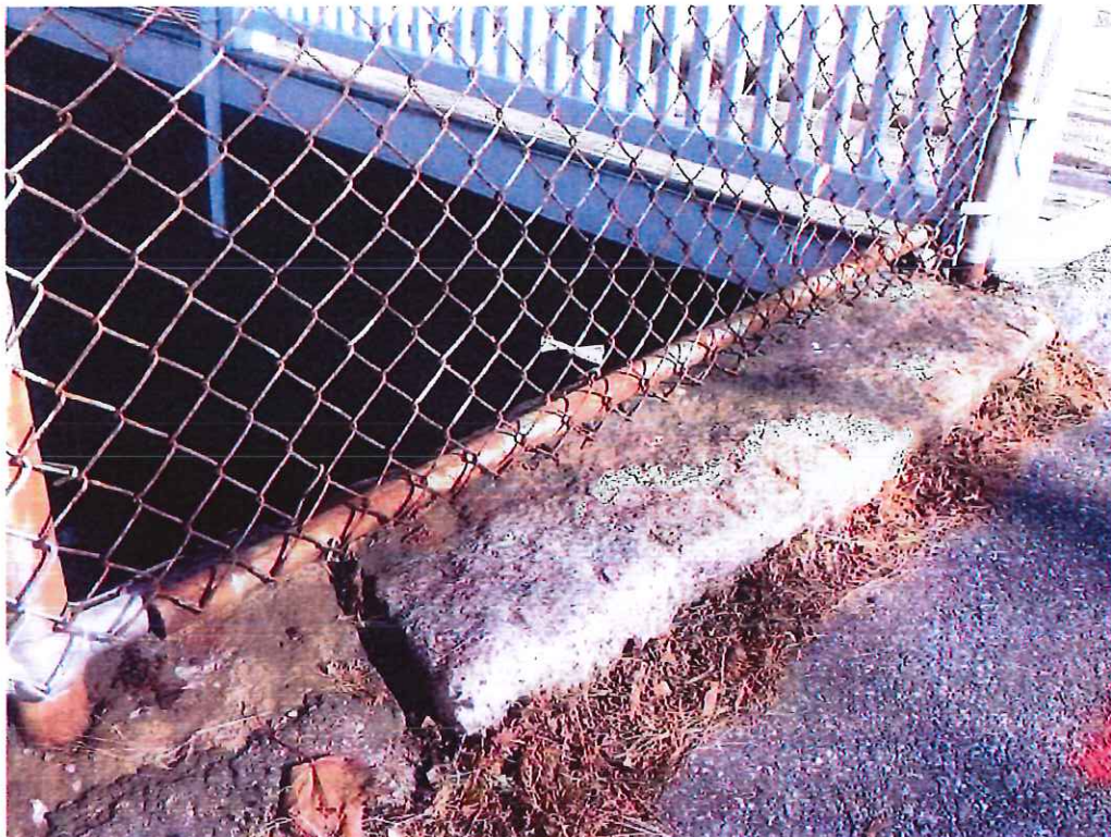
Photo 12: Railing - Northeast Panel: The bottom railing is detached from the receivers and hangs loosely.
