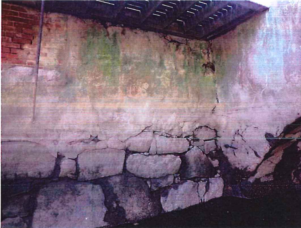
Photo 23: Wingwalls - Northeast Wingwall: Cracking and isolated hollow areas in shotcrete at the top of the stone masonry. Voids between stones up to 21" deep.
