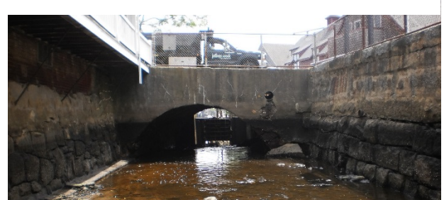
Photo 4: View of stream channel upstream from culvert looking south with dark staining on walls indicating normal high-water level when the gate is closed.
