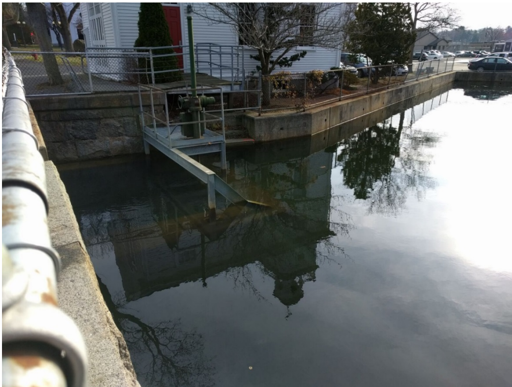
Photo 5: High Tide on December 3, 2017 the tide is well above the top of the tide gate
