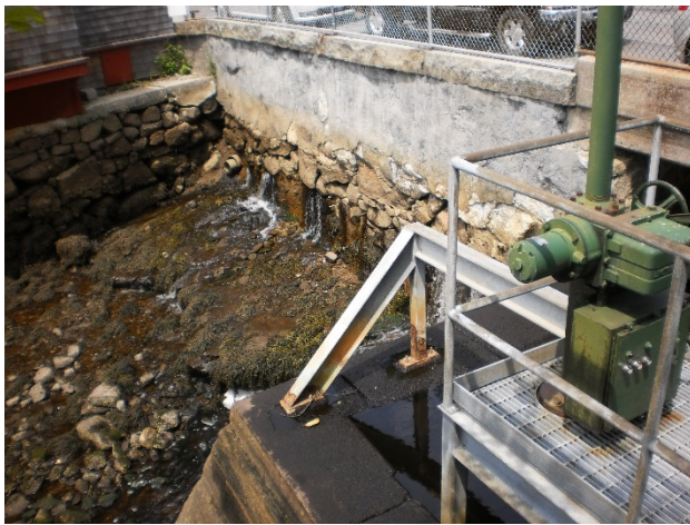
Photo 1: View of tide gate motor on the right and wall seepage on the left.
