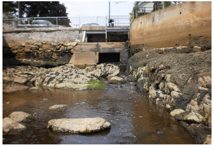
Photo 2: Looking upstream at the tide gate and Central St. culvert at low tide.
