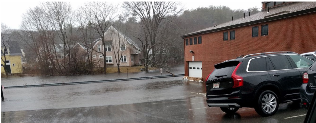
Photo 6: Central Pond adjacent to the Manchester Fire Department shown on 1/4/2018. Rising water levels eventually overtopped the wall (elevation 5.4 ft. NAVD88) flooding the parking area and Fire Department basement and garage area despite preventive sand bags across the door.
