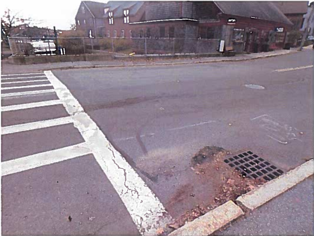
Photo 1: Moderate cracking throughout both lanes of wearing surface.
