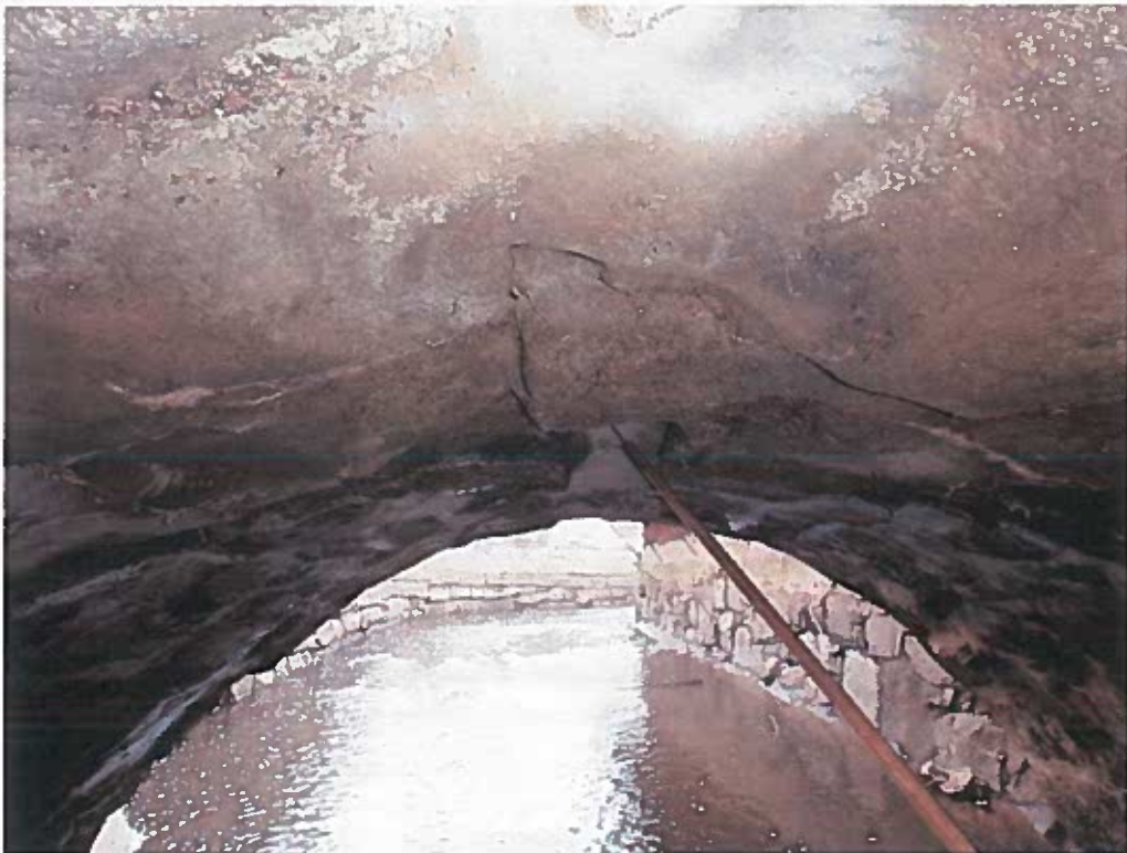
Photo 4: Keystone area with missing stones at north end.
