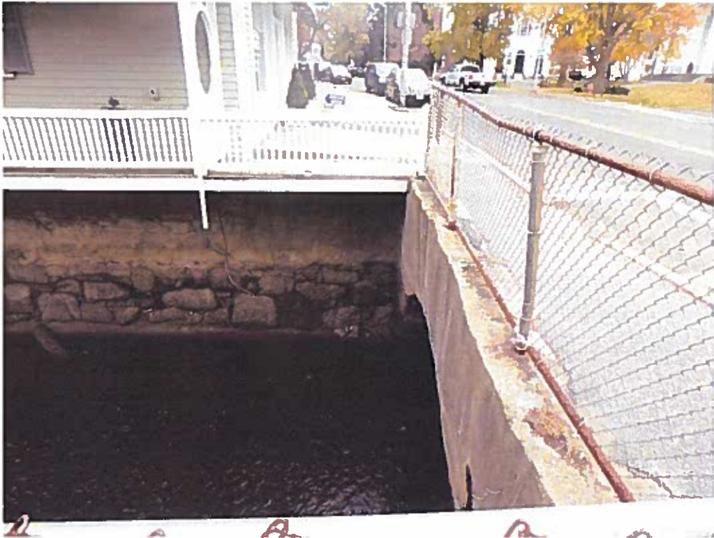
Photo 2: Corroded north rail and fence posts.
