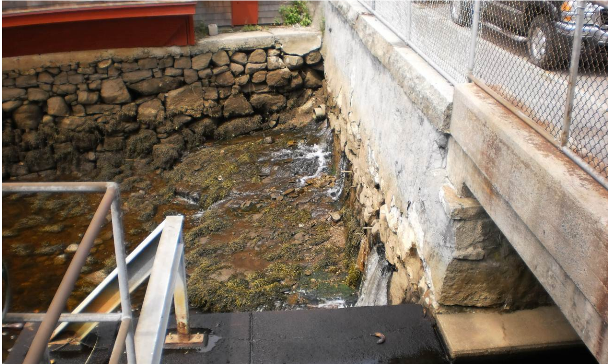
Photo 4 Water seepage (flow) coming from the stone culvert side wall
