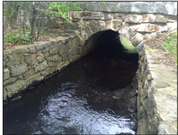
Sawmill Brook just upstream of its crossing of School Street near Brook Street.
