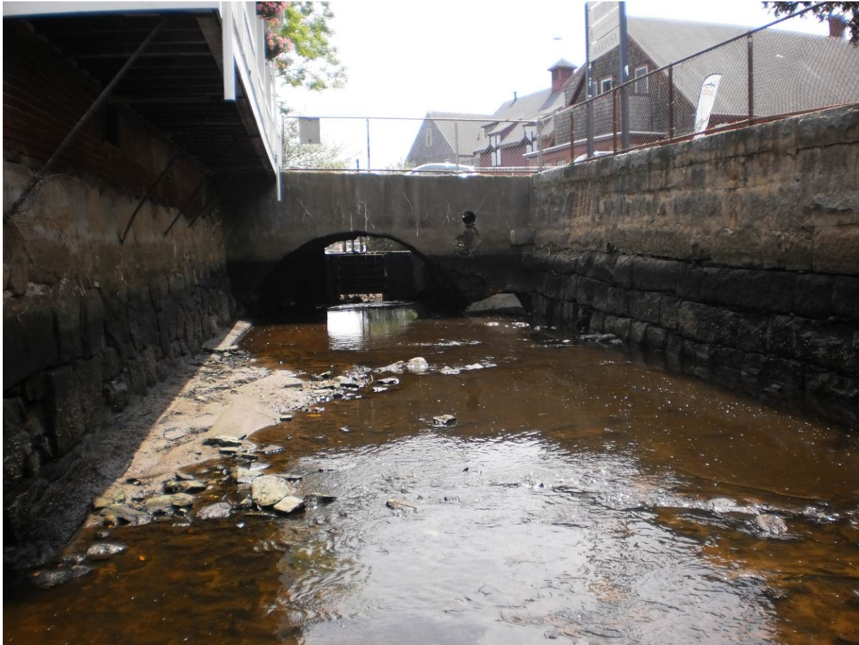
Photo 9 Stream channel upstream from culvert looking south with dark staining on walls indicating normal gate closed high water level
