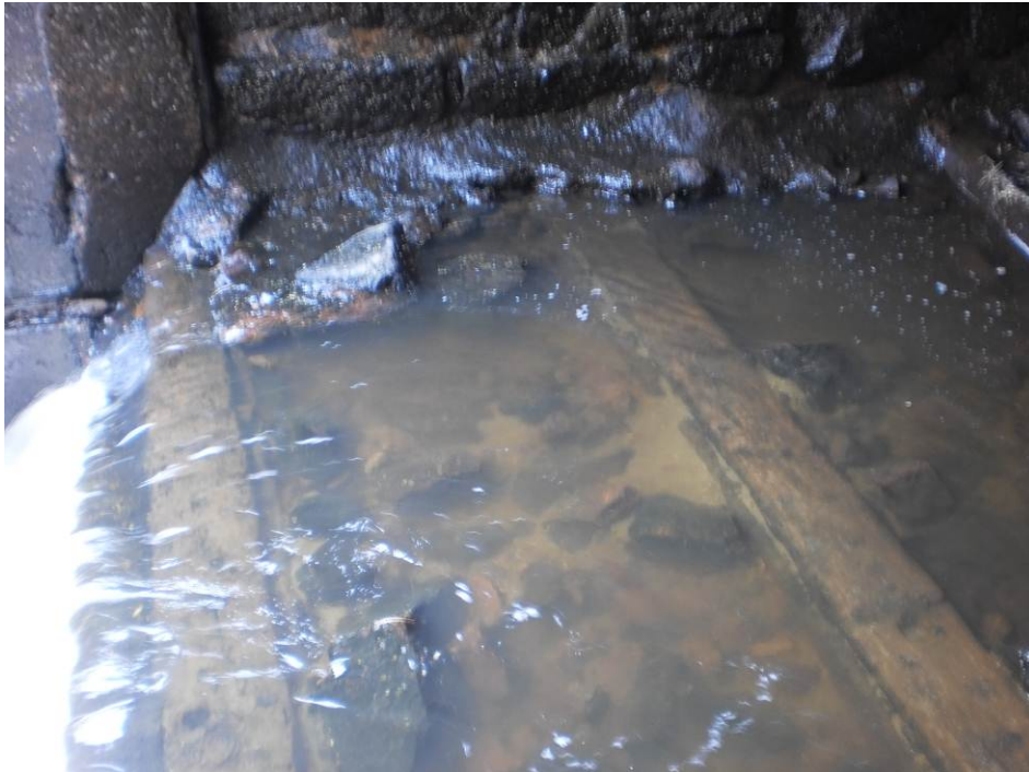
Photo 6 Apparent rock filled timber cribs forming stream bed at south end of arch culvert
