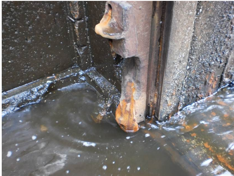
Photo 2 Corrosion/erosion of low tide gate tracks
