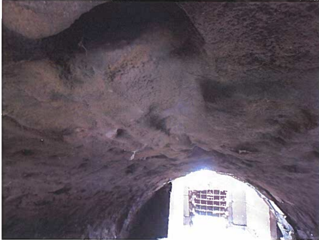
Photo 5: Missing keystone near mid-length with shotcrete patching, looking south.
