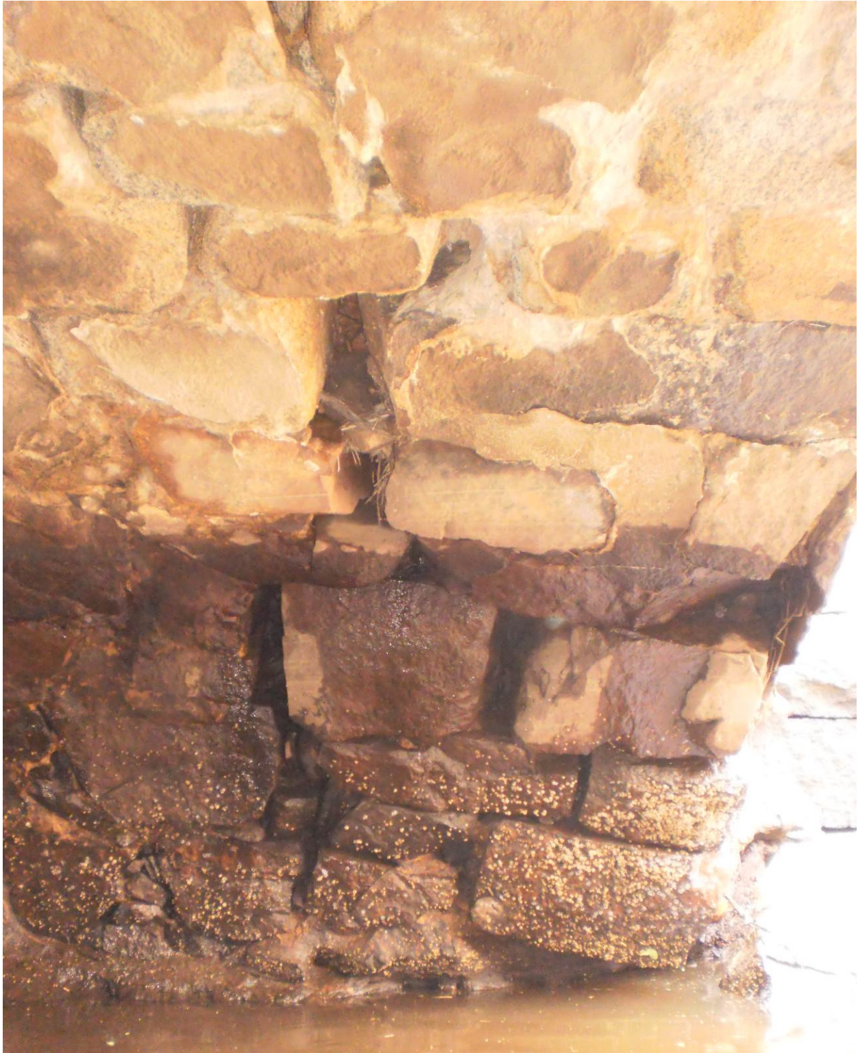
Photo 8 Separation and settlement of culvert arch stones, upstream, northwestern corner
