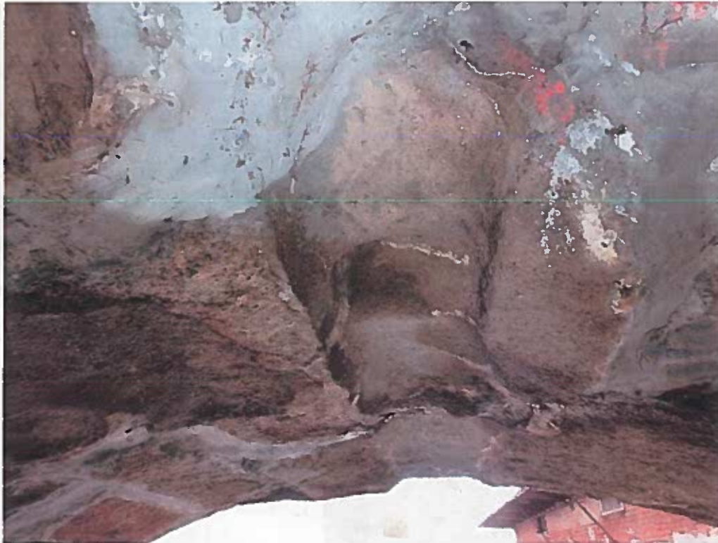
Photo 3: Keystone area with missing stones at north arch ring.
