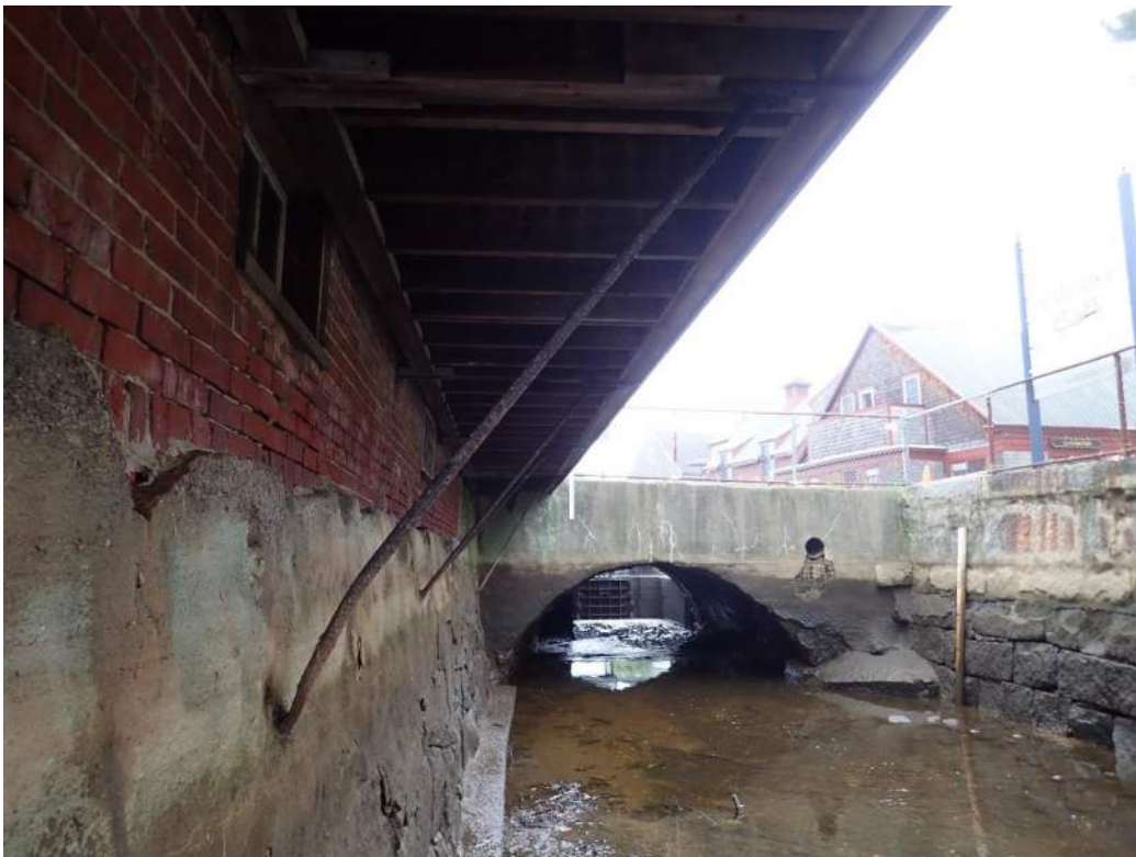
Photo 14: View looking upstream from the downstream side of the culvert toward the tide gate structure.
