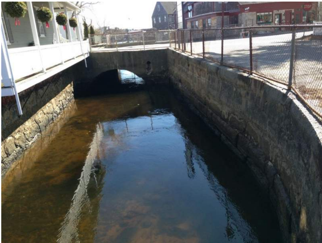
Photo 6: View of Central Street Bridge and approach channel walls from the south / upstream.
