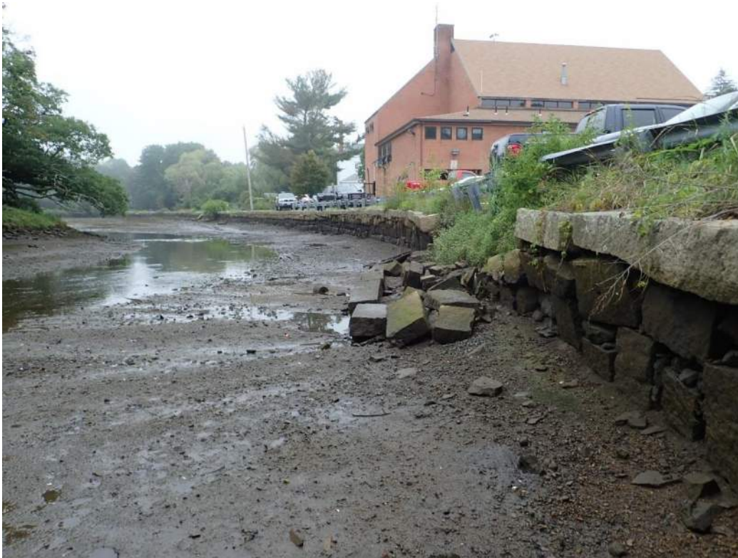
Photo 11: Deteriorated section of wall on the eastern side of Sawmill Brook / Central Pond, looking toward the Manchester Fire Department building.
