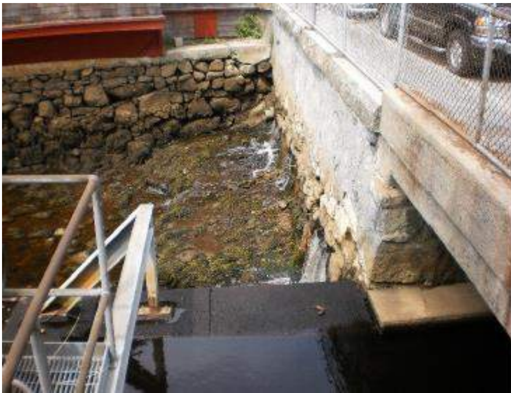
Photo 2: Seepage at the seawall from downstream.
