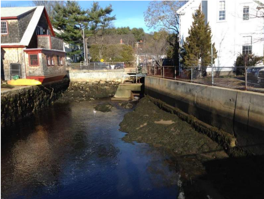
Photo 1: View of Central Street Bridge and tide gate from the north / downstream.
