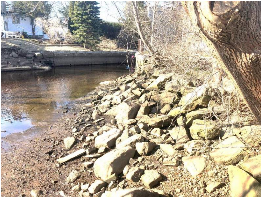
Photo 9: Transition from wall to riprap slope along Central Pond. Note collapsed wall on opposite bank.
