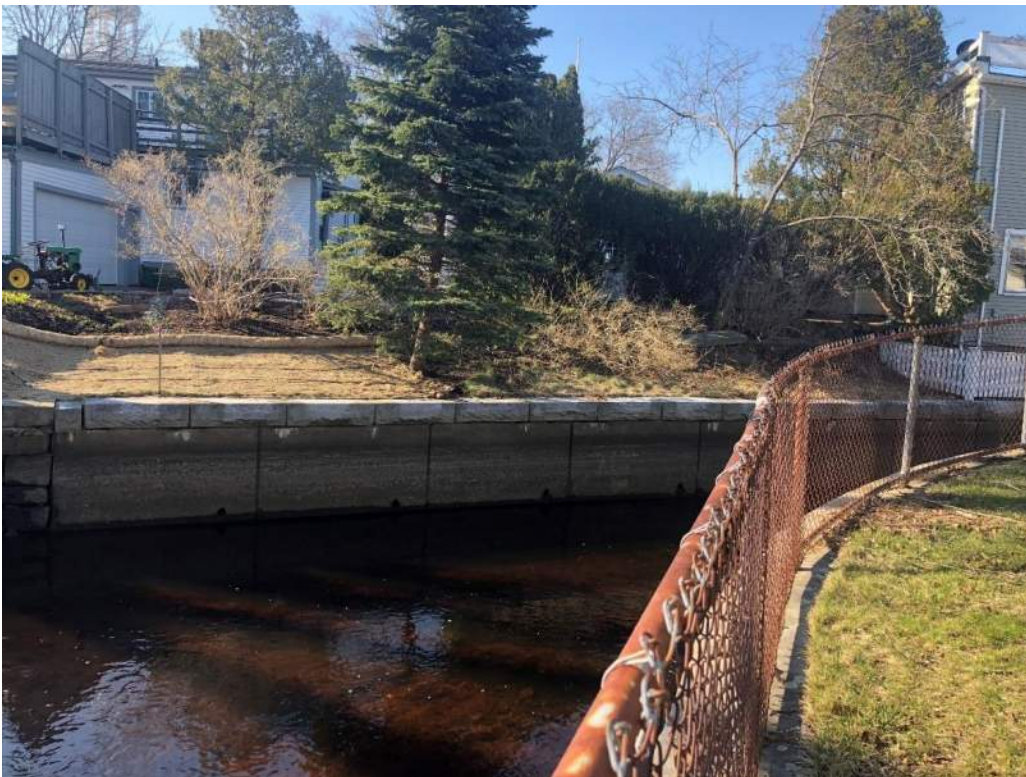
Photo 8: Segment of precast wall along Sawmill Brook between Central Street Bridge and Central Pond.
