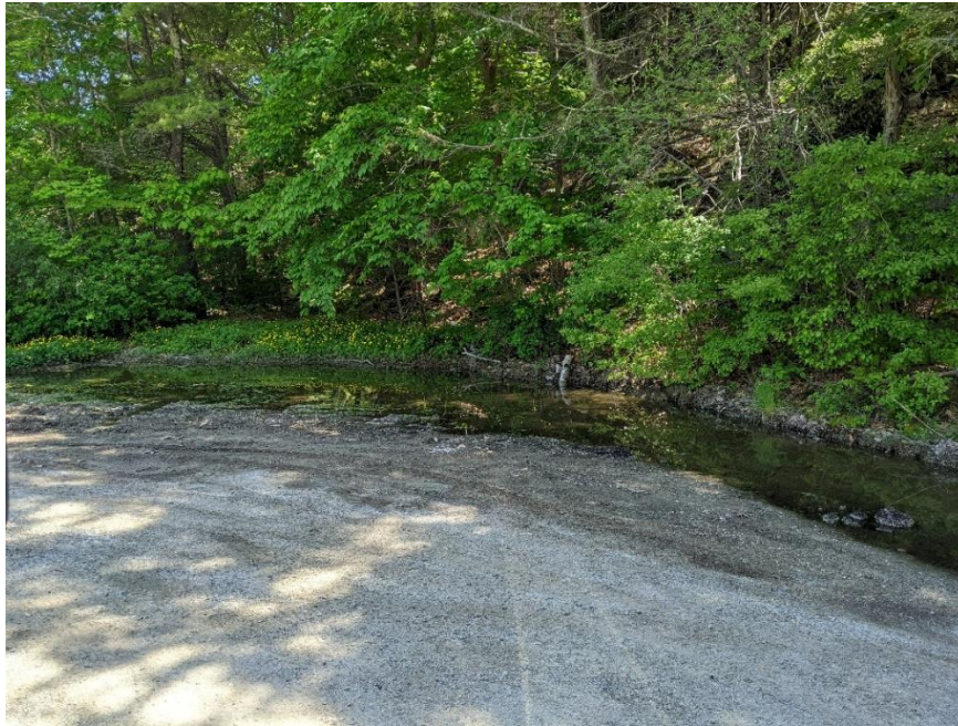
Stormwater is flooding the far end of the parking area at Sweeney Park.
