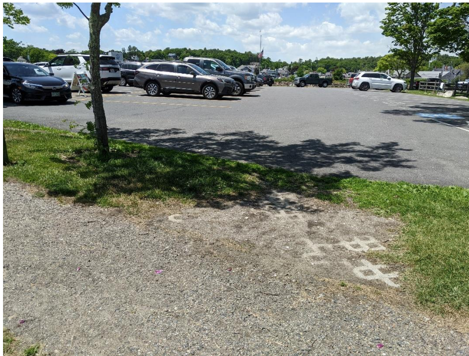
There are two low points where stormwater flows off the pavement. The permeable paving is compacted with sand and gravel.
