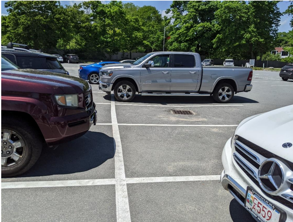
Stormwater runoff collects at one catch basin in the middle of the parking lot where sand from the beach is also being washed away.
