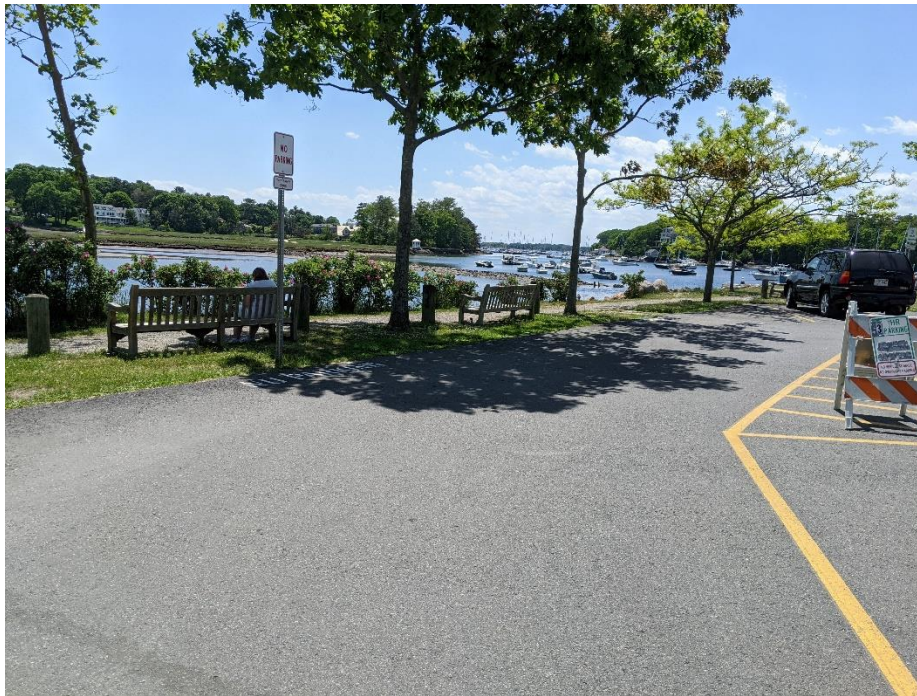
The paved parking lot at Masconomo Park is located adjacent to Manchester Harbor, where runoff directly discharges.
