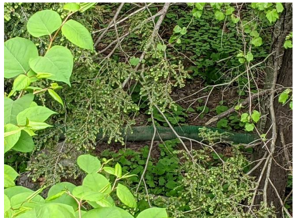
4. Dirty erosion sock from turbidity of runoff
