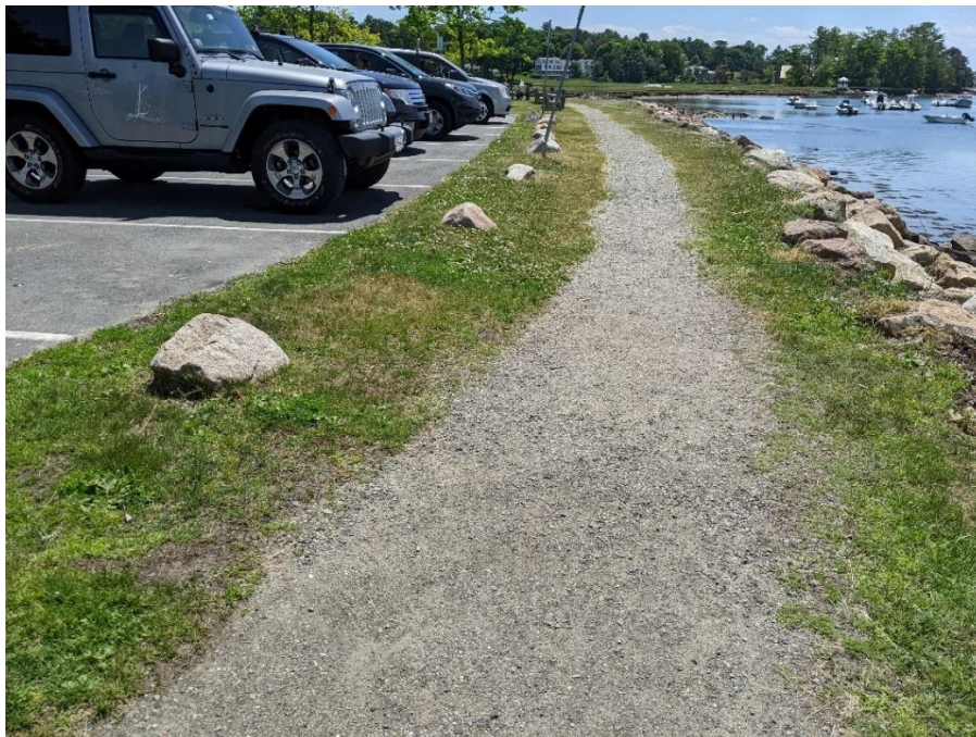
Rip-rap could be extended to help prevent bank erosion.
