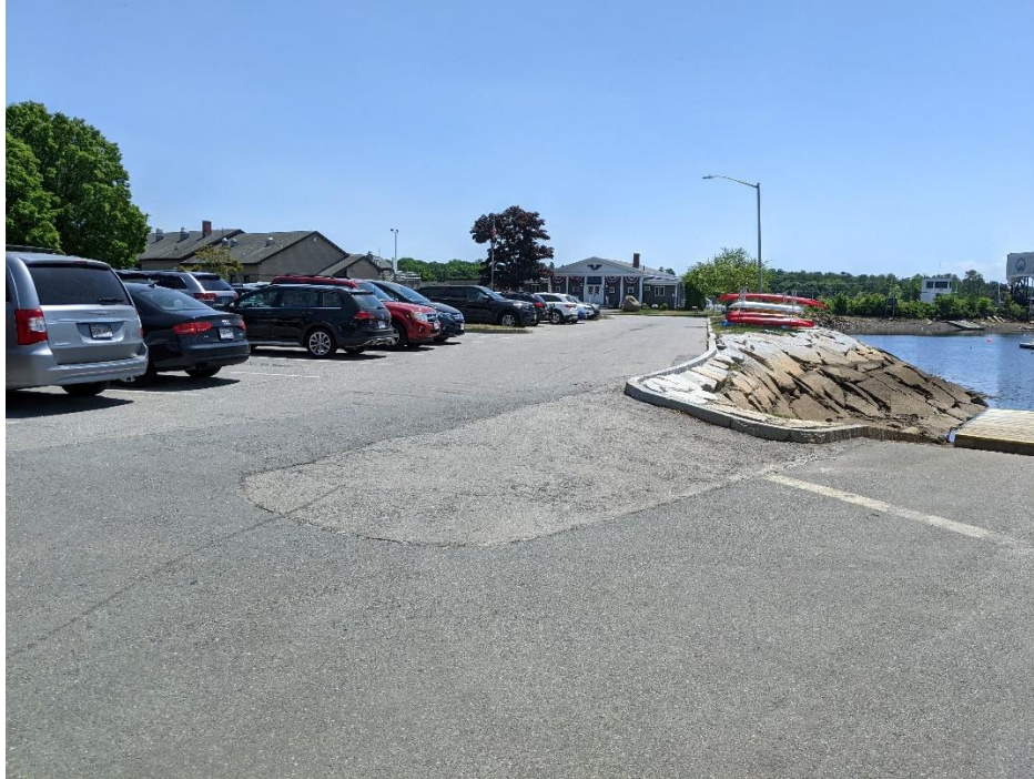
Parking lot catch basins drain to two outfalls that discharge directly to Manchester Harbor.
