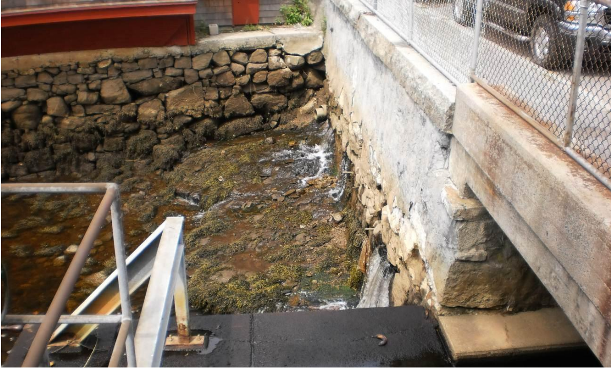
Water seepage (flow) coming from the stone culvert side wall
