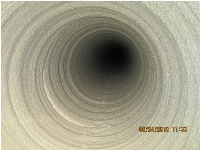
Cement Lined Water Main
