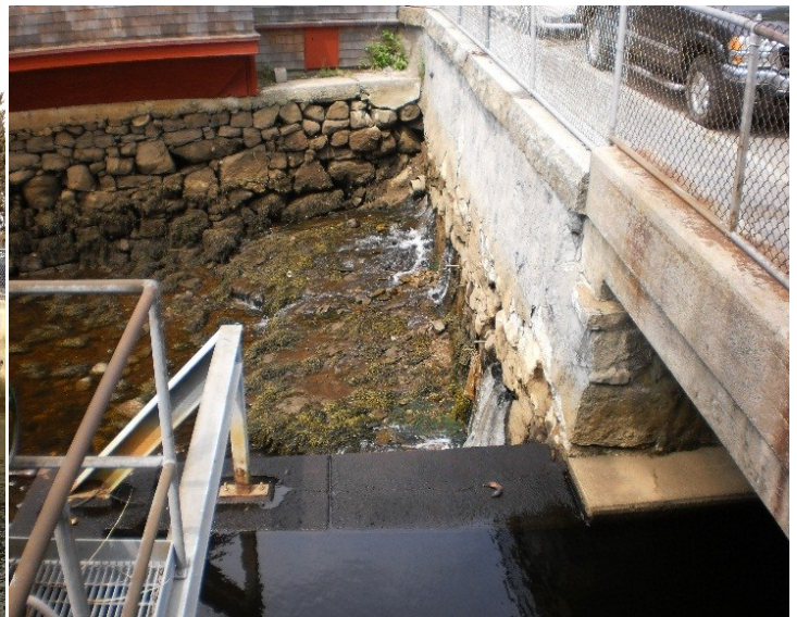
Seepage at the seawall.
