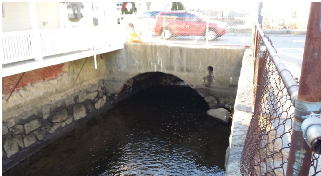
Storm drainage from Central Street with direct discharge to Sawmill Brook
